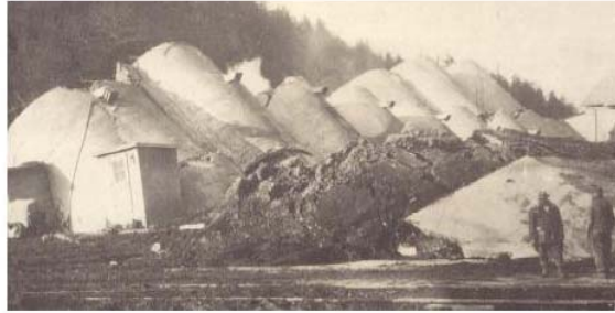
Figure 5-2: Bearing Capacity Failure of Silo Foundation (Vesic, 1975, from Tschebotarioff, 1951)
